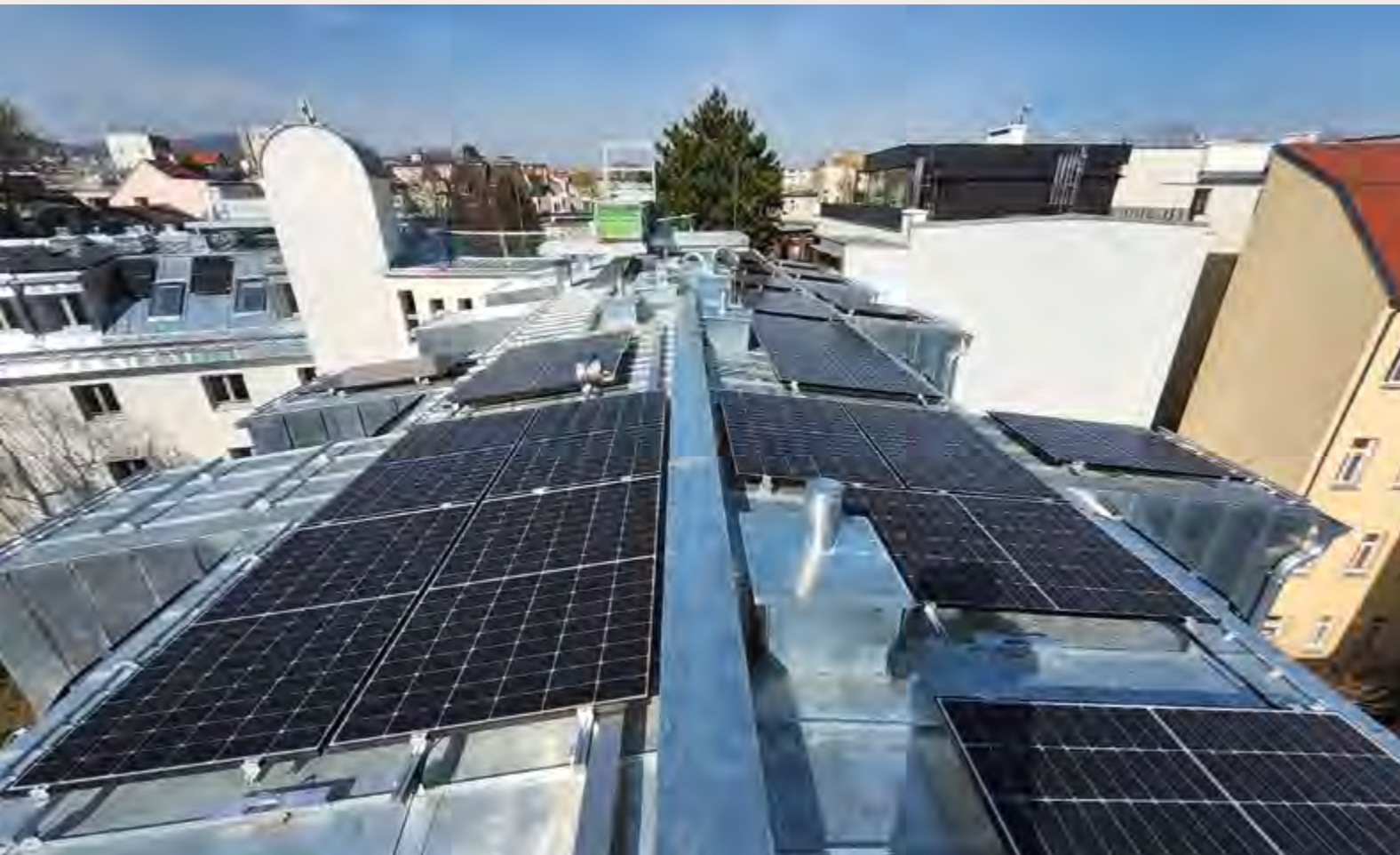
☛ Photovoltaik am Dach
